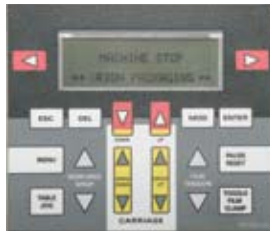
Control Panel HMI
